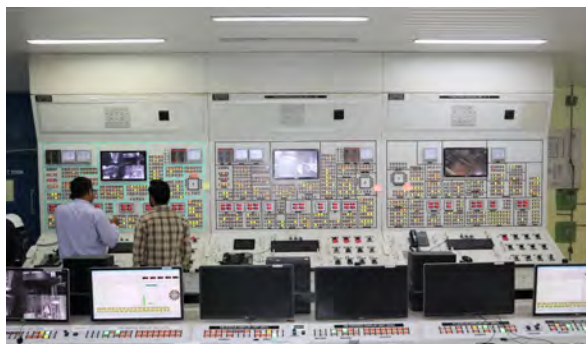
Fuel handling control panels
