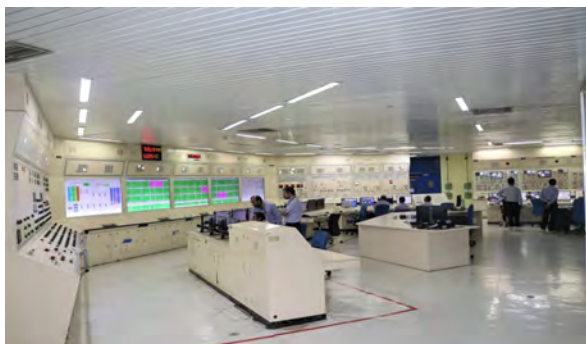
Main Control Room
