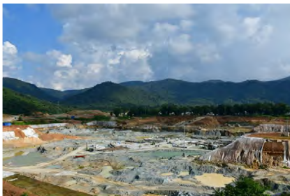
KGS-5&6 Main plant area
